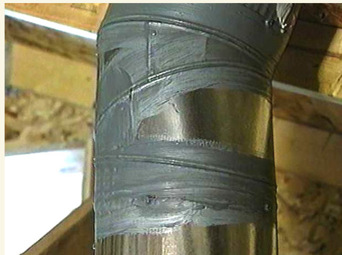
Properly Sealed Duct
